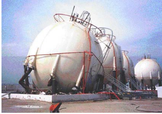
Figure1. Failure of welded structures
